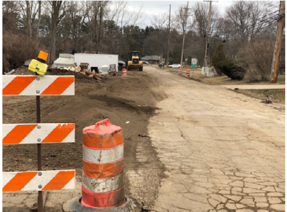
Work continues on the water main replacement and street paving project in Washington Village neighborhood in the vicinity of Northwestern Highway and Nine Mile. Due to mild weather, work continued on this two-year project throughout most of the winter. The result will be an earlier completion date in 2020.
